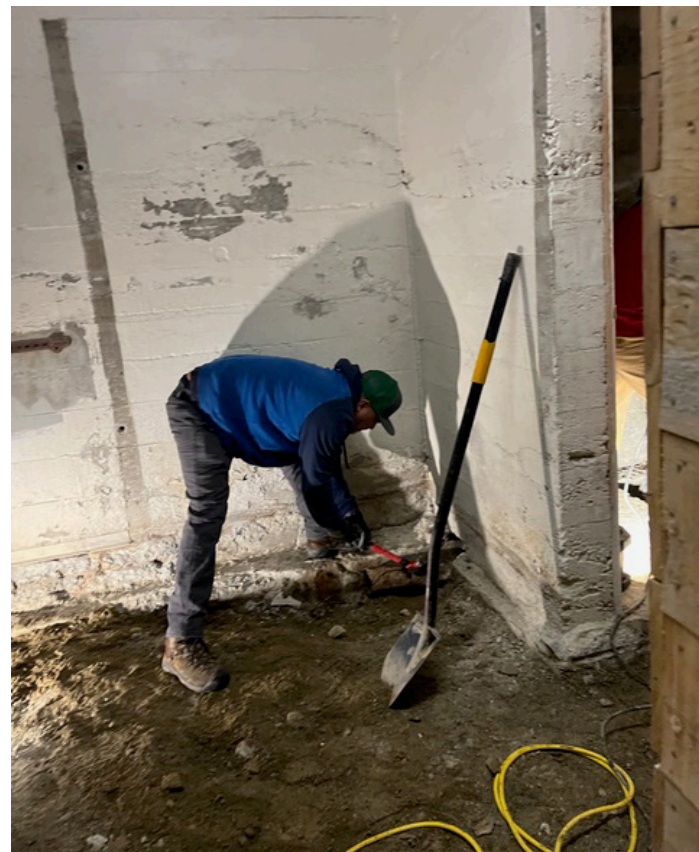
The first phase of the renovation includes repairs and updates to the basement of the Grange Hall, including updating a 75-year old sewer line and modernizing and making the restrooms accessible.
